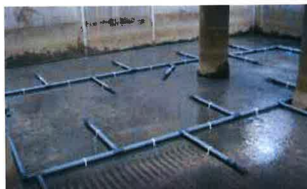
ASBS circuit clipped and completed in an underground tank. Note: vale at pier fitted at 45 angle to avoid dead spot
